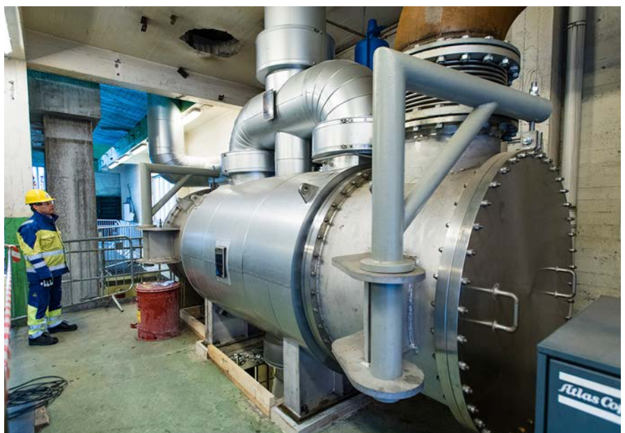
The upgraded energy recovery plant at Bjølvfossen.
